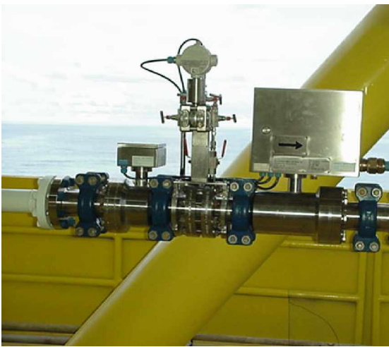
Fig. 4 Photograph of ESMER T3A installed at SFJT – C offshore platform
